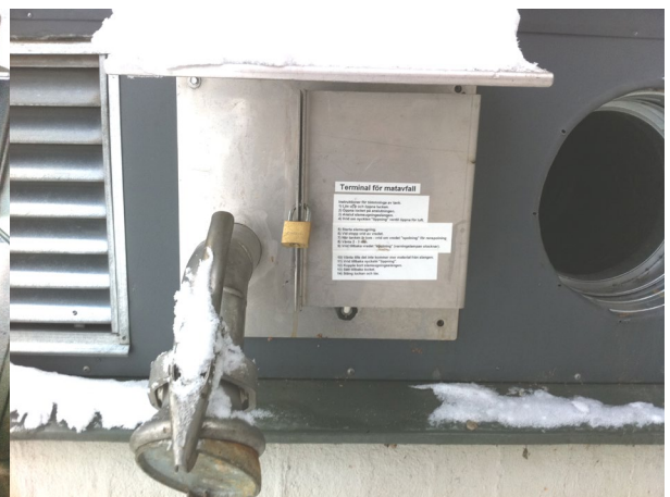
Terminal for extraction truck
